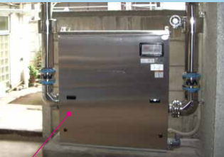
Direct connection water supply booster pump
