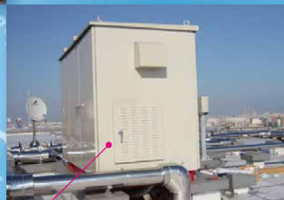
Cubicle type fire pump
