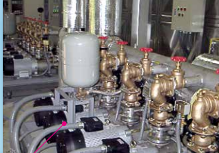
Pressurized water supply pump
